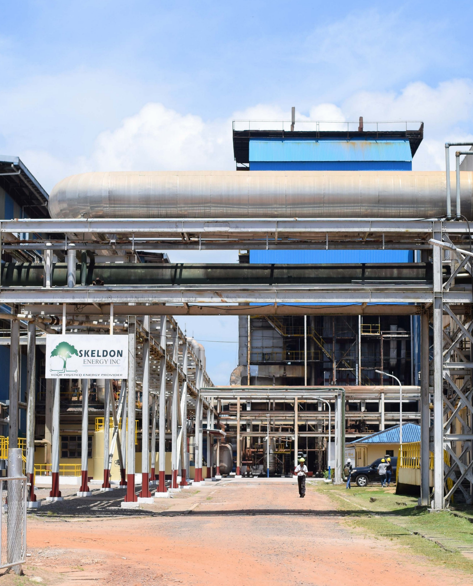
The Skeldon Estate Co- Generation Power Plant. | Photo compliments: DPI Guyana
