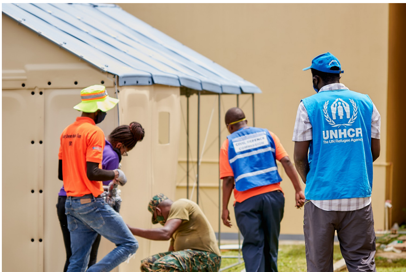
Staff from the Civil Defence Commission and UNHCR working together to set up the pre-fabricated housing units at the Mahaicony Hospital, Region 5 which serve as isolation-quarantine facilities.
