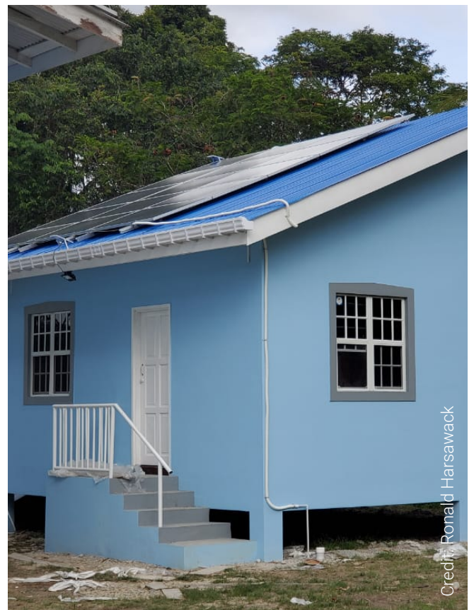
15 panel array 5KW photovoltaic system installed at Bethany Essequibo Coast, Region 2, Guyana.
